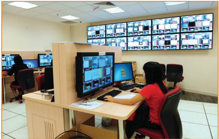
Figure 5 The control room at Nanyang Technological University
